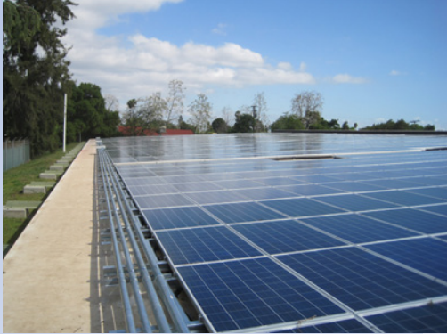
Installation of a solar array (shown here) in Pasadena is one of the ways NASA is optimizing the cleanup process.
