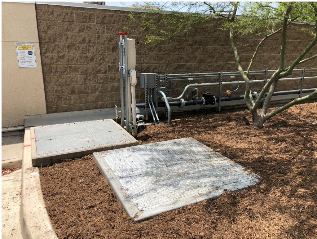
Figure 5-2. Above Ground Piping and Conduit Behind JPL Fire Department (Includes New Utility Vault)
