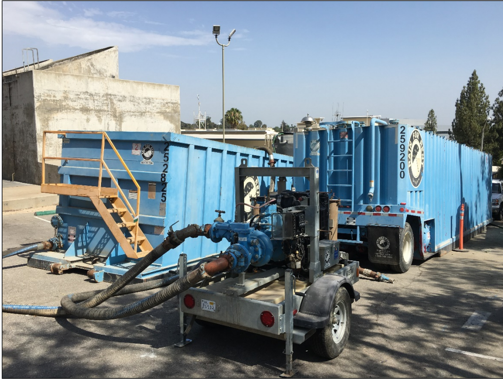
Figure 4-1. Temporary Treatment System
