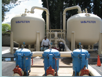
Ion exchange section of the Lincoln Avenue Water Company treatment system.
