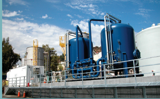
OU-1 Treatment System
