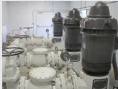
New pumps are shown at a booster station near the Ventura well, one of four previously closed and now upgraded wells in the Arroyo Seco. Image Credit: NASA/Battelle
